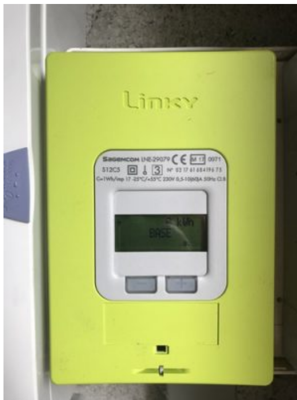
Figure 1. Linky meter. [Source: © Benoît Prieur / Wikimedia Commons]
