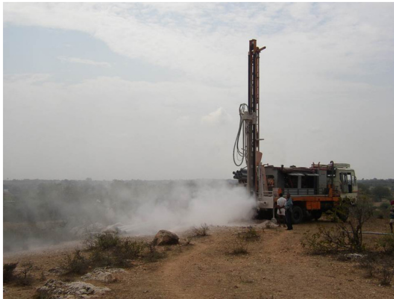
Figure 3 . Drilling in progress in a granitic aquifer using the "down the hole hammer" method. Kothur, Andhra Pradesh, India. [© B. Dewandel]
