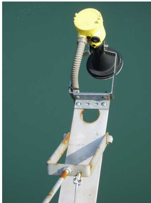
Figure 5. Level measurement by emerged radar. [© EDF DTG]
