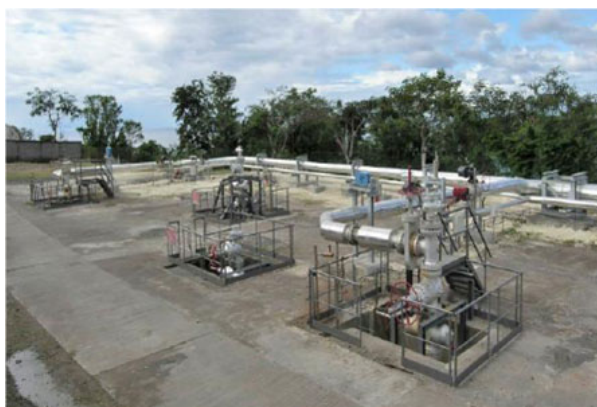
Figure 4. View of the production wellheads of the Bouillante field on the island of Guadeloupe. [Source: photo CFG services]
